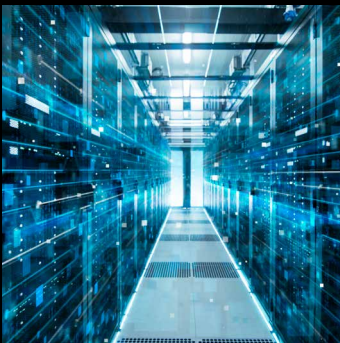
Networking and IT Infrastructure
