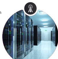
Data Center Smoke/Water etc Sensor
