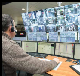
Sale comando e control room
